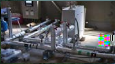
The geothermal heat pump experimental system
